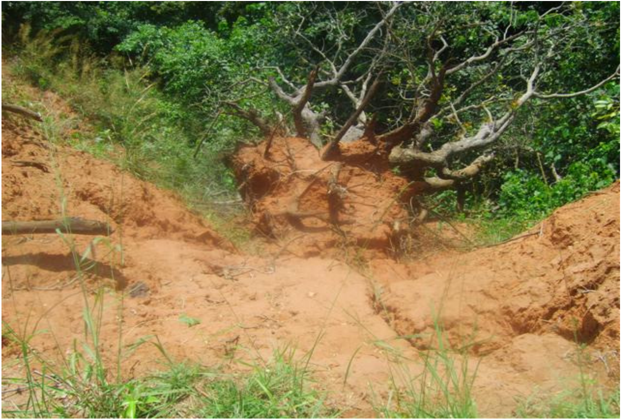
Figure 5 Erosion site at Agu-Ukehe road, Amadim (Photo by Ani U. A. Nov. 2008)
