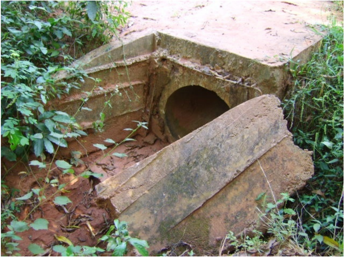
Figure 23 Umuoda Lejja erosion damaged drainage canal (Photo by Ani U. A. Jan. 2009)
