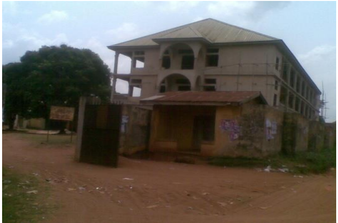
Front view of St. Theresa's College building Obollo. Many students from Ehime and Isu area attend the school which is an avenue for inter/intra human interactions.
