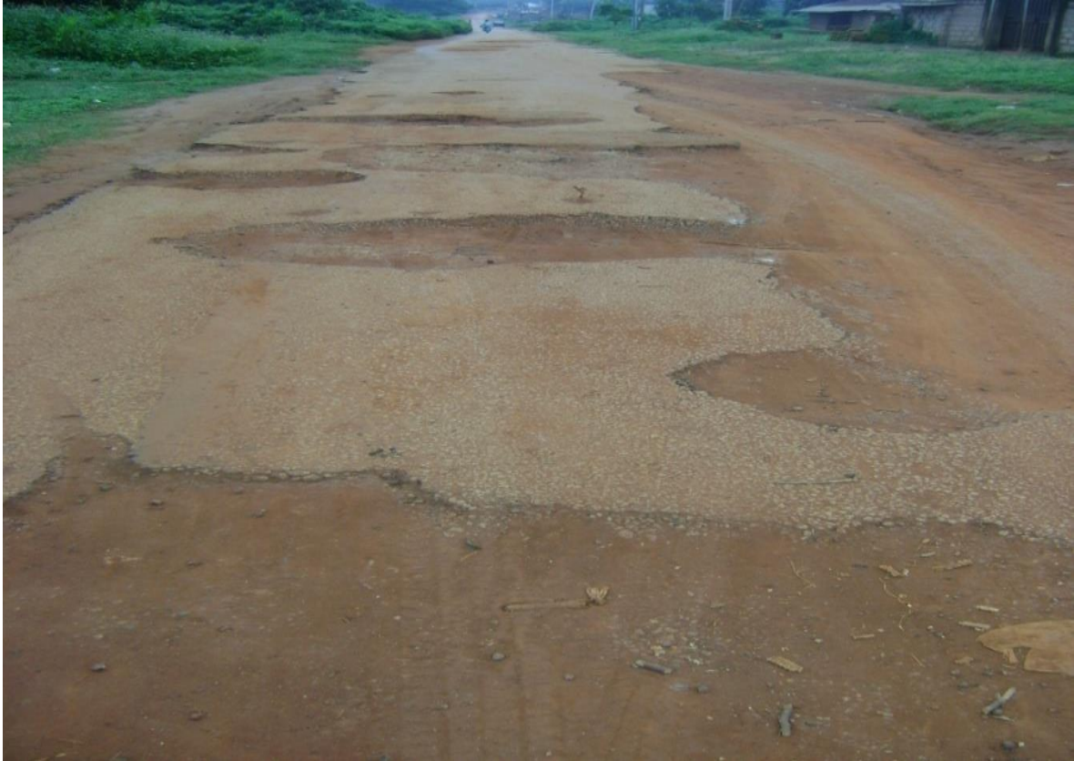
PLATE 8: This picture is showing the part of the Opoji old road where the profile was taken.
