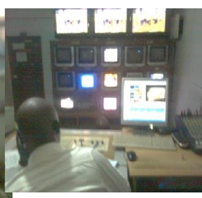
(g) Master control room
