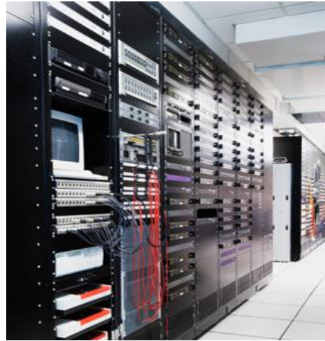
(a) Equipment racks
