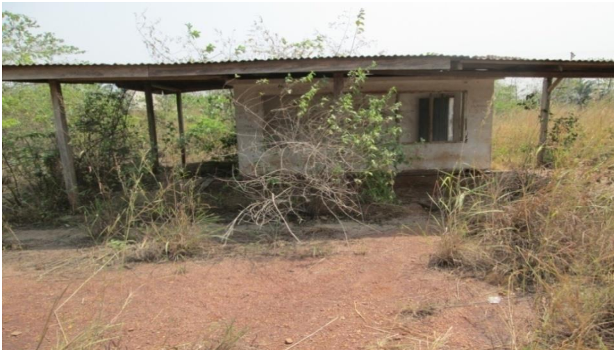
Plate: 6 the ancient building at Enyigba mine, (built by British miners in 60s)
