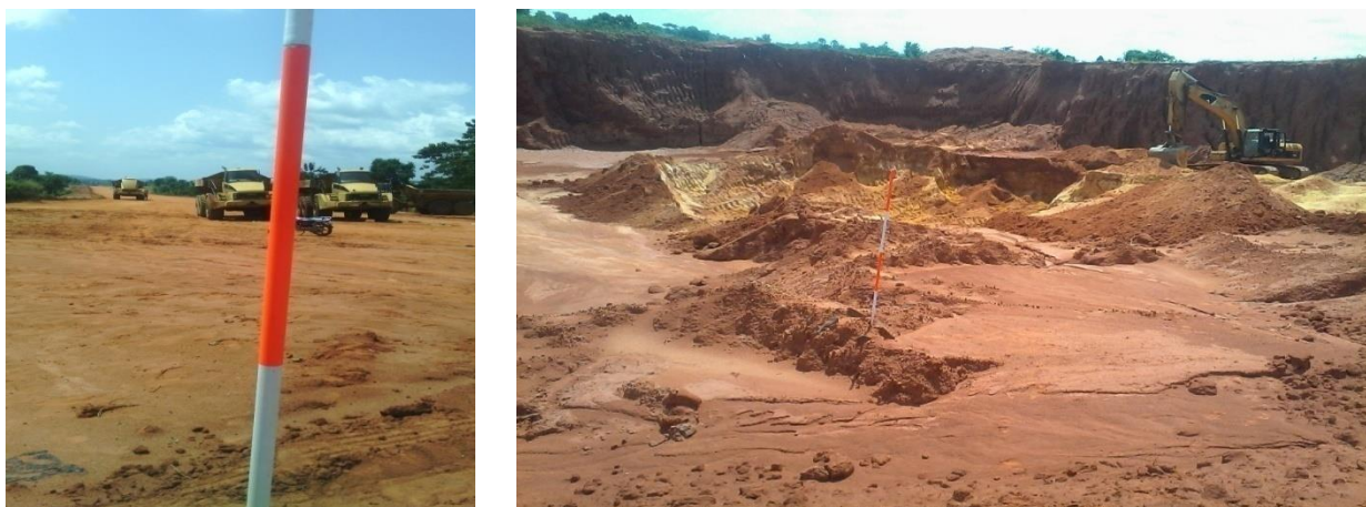
Plate 7: Link Road and the Borrow Pit at Ifite-Umueri Axis
