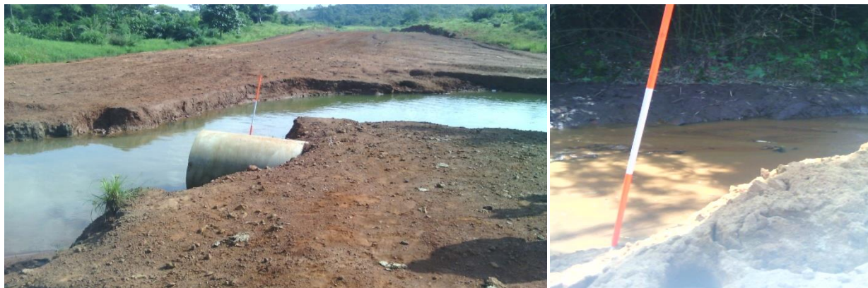
Plate 9: Destruction of Iyi Ogene at Nenyi axis in Umueri and Kpeke Stream at Ifite Axis of Umueri; the Community Source of Water
